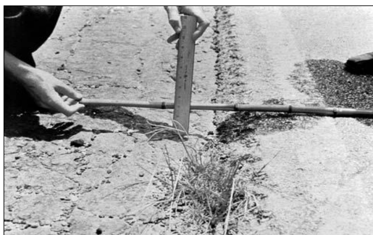
FIGURA 52: Severidad Medio (M) Desnivel Carril-Berma. FUENTE: American society for testing and materials, 2018.
