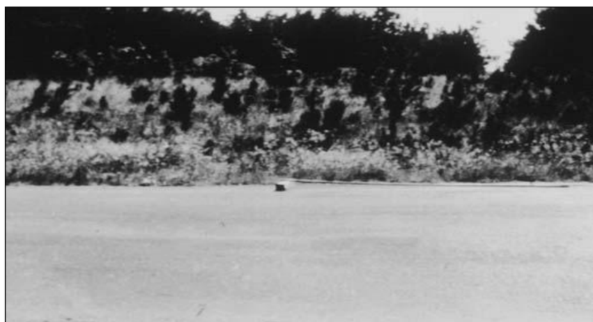
FIGURA 73: Hinchamiento. FUENTE: American society for testing and materials, 2018.
