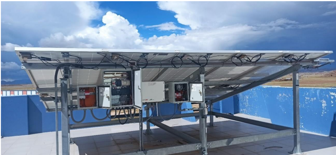
Figure 8 Installation of the SFCR Solar Edge data acquisition system.
