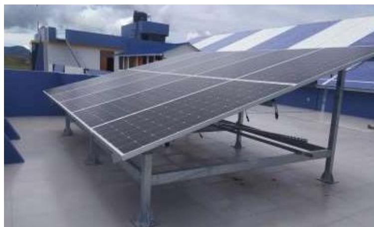
FIGURE 1 SFCR installation with Solar Edge inverter and CC-CC optimizers.
