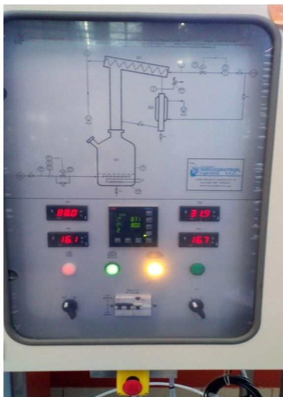
Figura 6: Panel de control.
